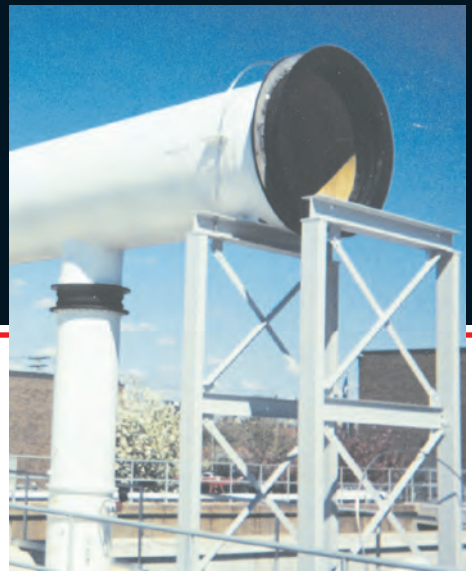
Redflex® circular 48-inch ducting joints on a large-scale aeration system.
