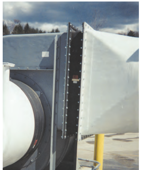
Blower system using 60-inch rectangular and 60-inch round ducting expansion joints.
