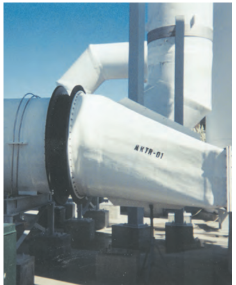
Circular 72-inch ducting joints on an air recovery system at a coal-fired power plant.
